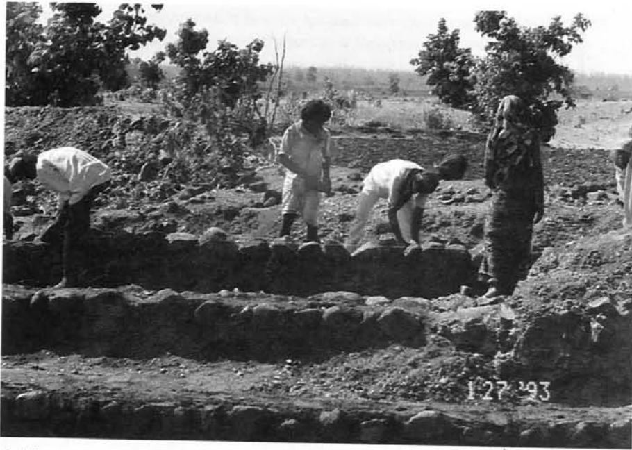
Rubble masonry work to strengthen an earthen dam in a village in Dewas district
