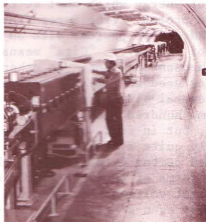
A view inside the tunnel of CERN's Super Proton Synchrotron (SPS). This accelerator has a diameter of 2.2 kilometres and achieves a proton energy of 400 GeV.
